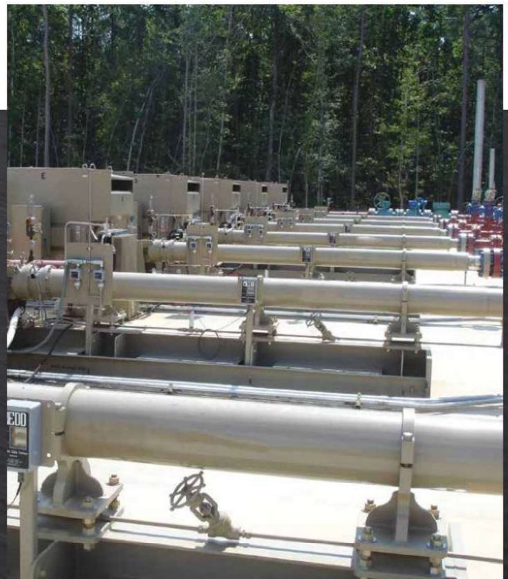
CO 2 pipeline booster (North America)
