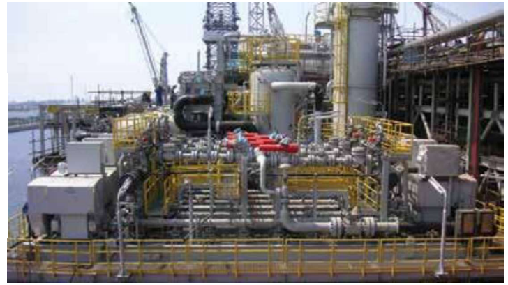
FPSO treated sea water injection (Africa)
