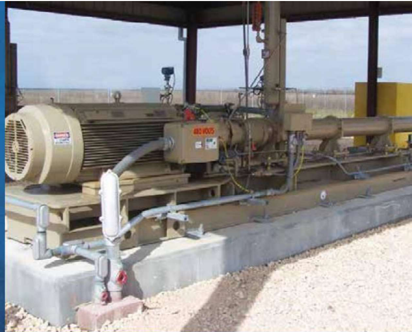
Ethane pipeline booster (North America)
