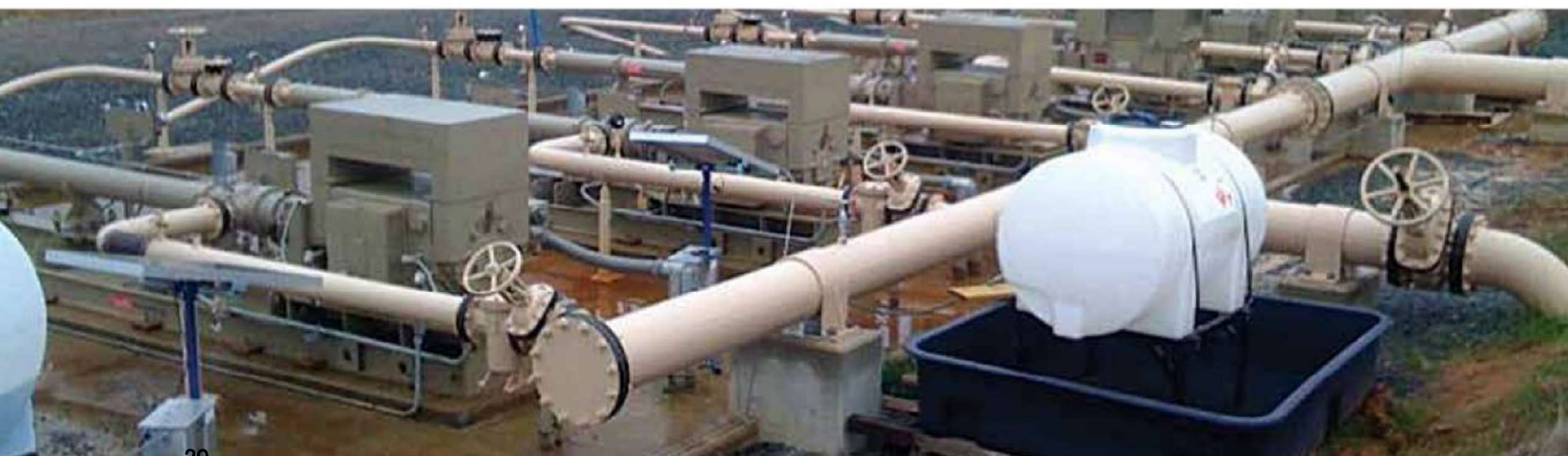
Water transfer installation (North America)
