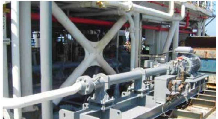
FPU crude oil transfer (Gulf of Mexico)
