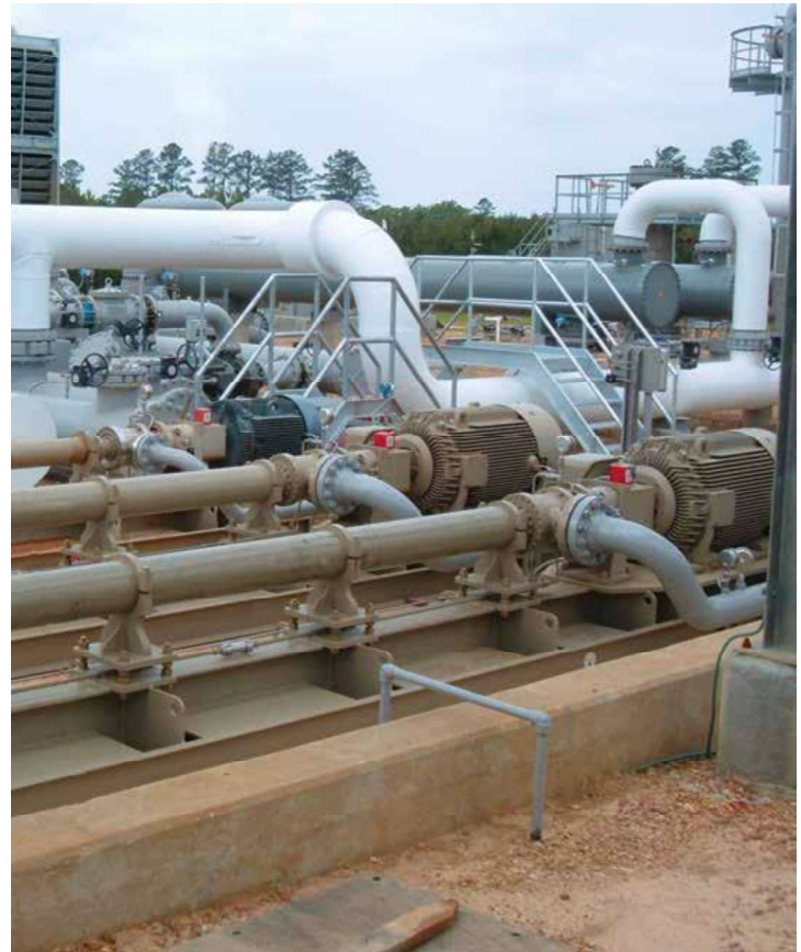
CO 2 pipeline booster (North America)
